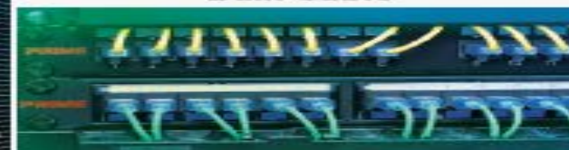
Patch Cables & Panels
