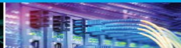
Fiber Optic Cables
